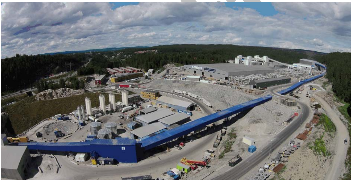
Installation area Folloline, NO
